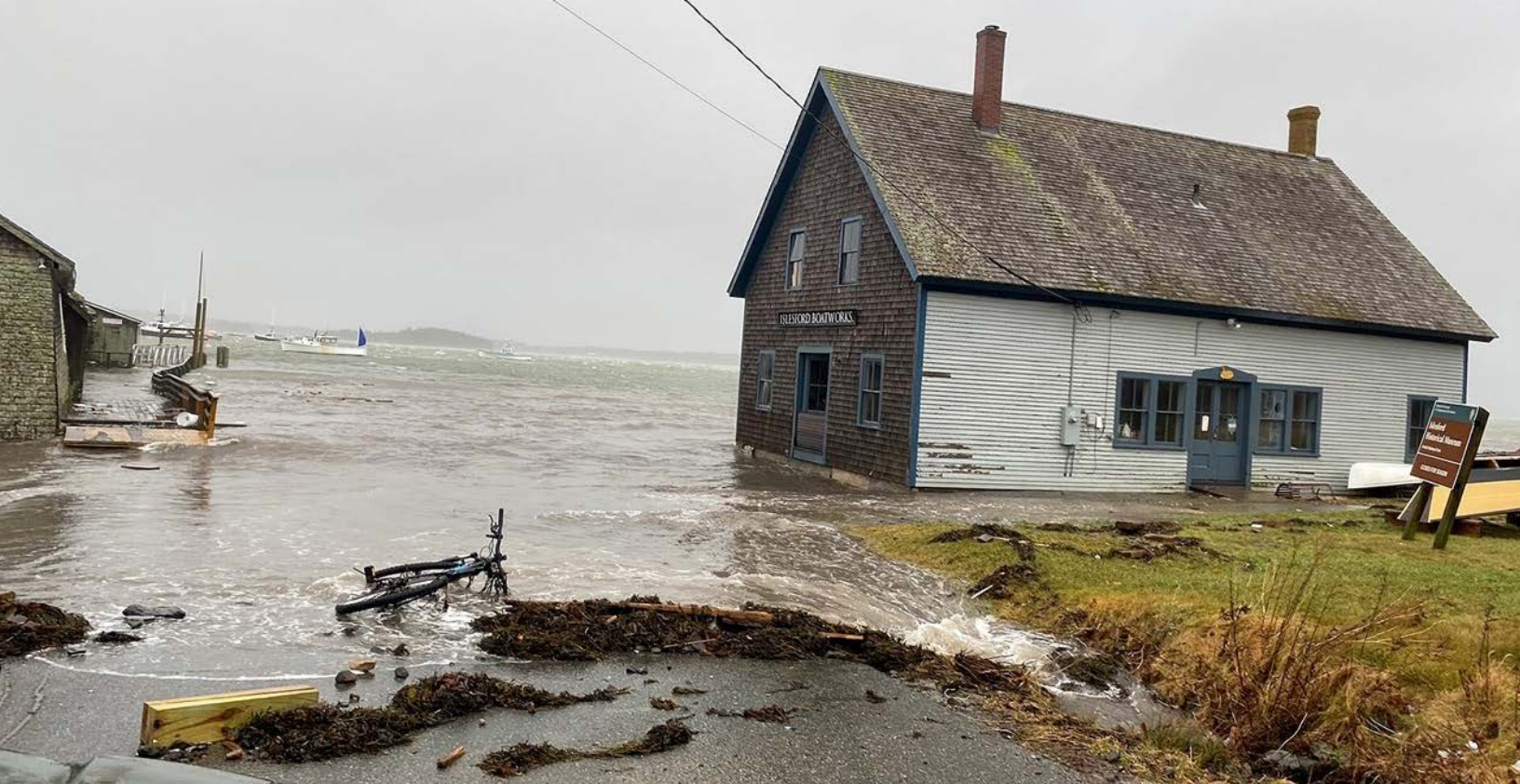
Storm damage to the Blue Duck Ships Store, Acadia National Park | Photo: Melissa Amuso NPS
